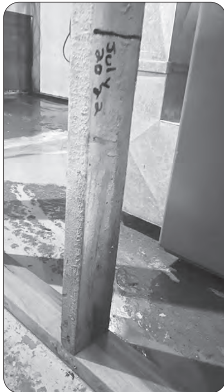
Marks on this post indicate how high the water rose in Patty Kowalchuk's basement.
