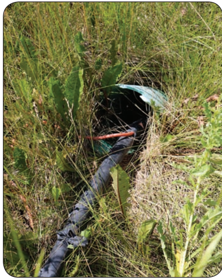
Rockwood residents would like to see open wells, seen above, on quarry property capped to avoid future contamination.
