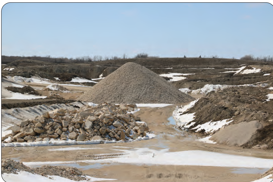
A mountain of material is shown here in April, piled up in one of the rock quarries north of Stonewall.
