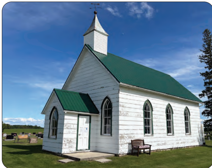
Victoria United Church, built in 1883 in the Victoria district south of Balmoral, is the focus of a new $65,000 capital campaign aimed at preserving the historic landmark through critical exterior restoration work.
