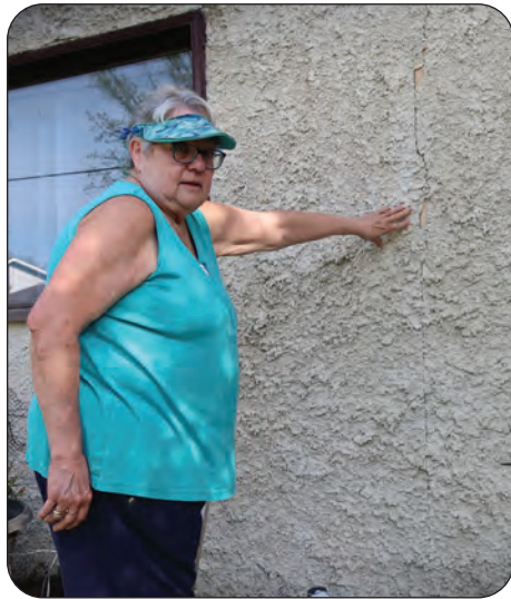
Vi Dueck points to cracks in the stucco on her Stony Mountain home.
