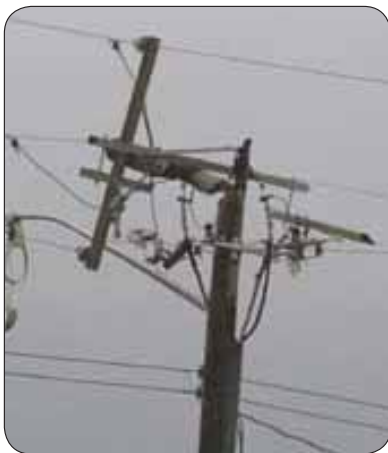
Excess dirt around the insulator was the cause of the pole fire last Thursday.
