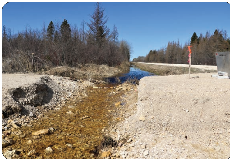
Runoff took out Road 9E at 124 NE in the RM Armstrong. Photo taken April 28.
