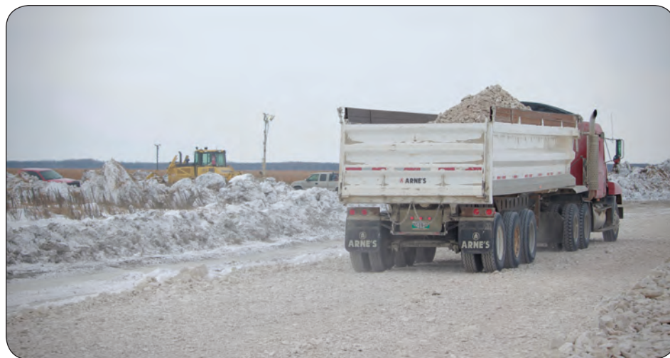
The province expects all work to be completed later this spring, but it's dependent on weather.
