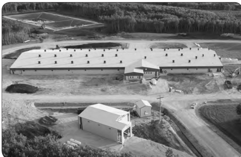
The company's Delta Canada facility will house around 2,600 animals and test 7,500 nucleus boars in the company's TN Tempo sire line and Z-line dam line every year.
