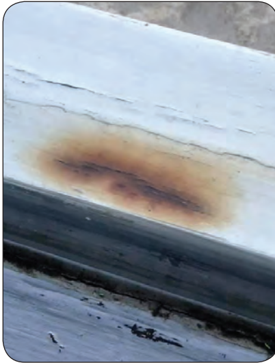
The charring on the windowsill is what the Keeley family suspect to be the lightning's exit point.
