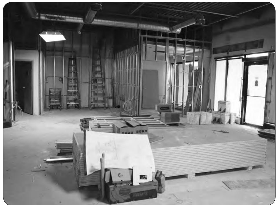
TRIBUNE PHOTO BY JO-ANNE PROCTER Stonewall's south end mall is under construction. The mall is scheduled to open this fall with a medical clinic and optometry clinic.
